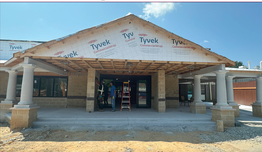
July 22, 2025. Electronic sdoors are installed in the new Welcome Center.
